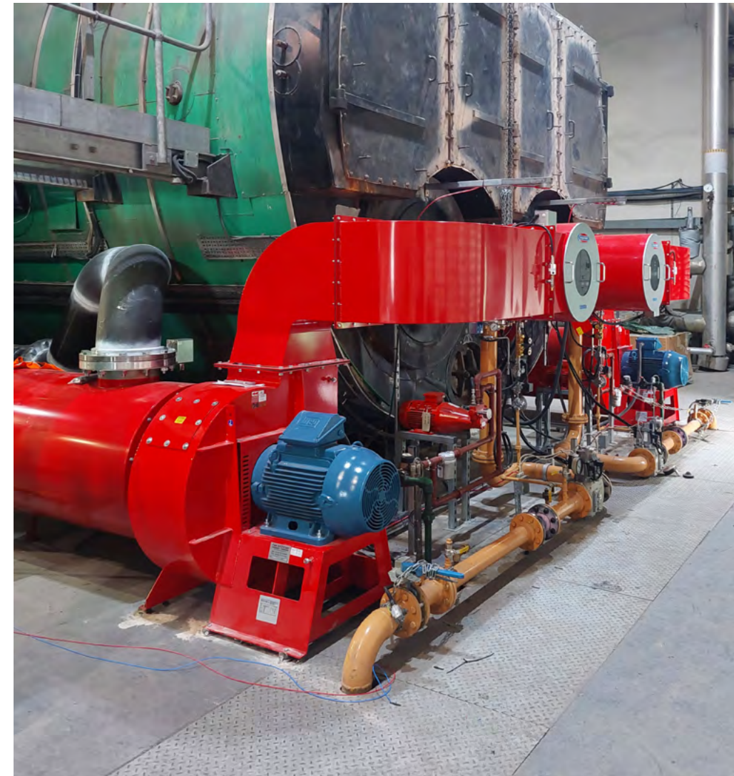
Picture of the newly installed burners in Pollington, which save us up to 600 tonnes CO 2 annually.
